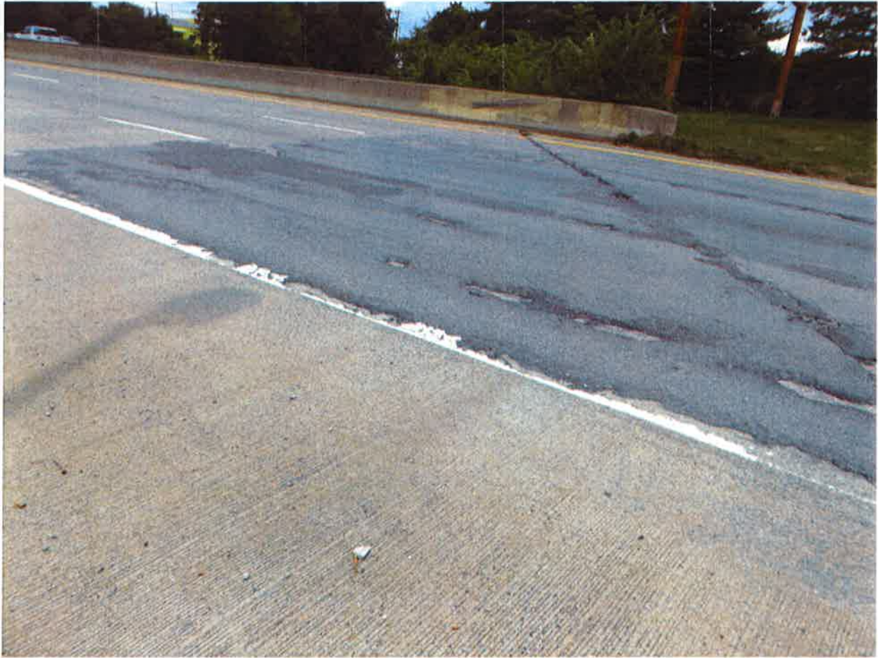
Pic #42 Approach 2 and part of the Bridge @ Abut. 2 is covered w/ Asphalt
