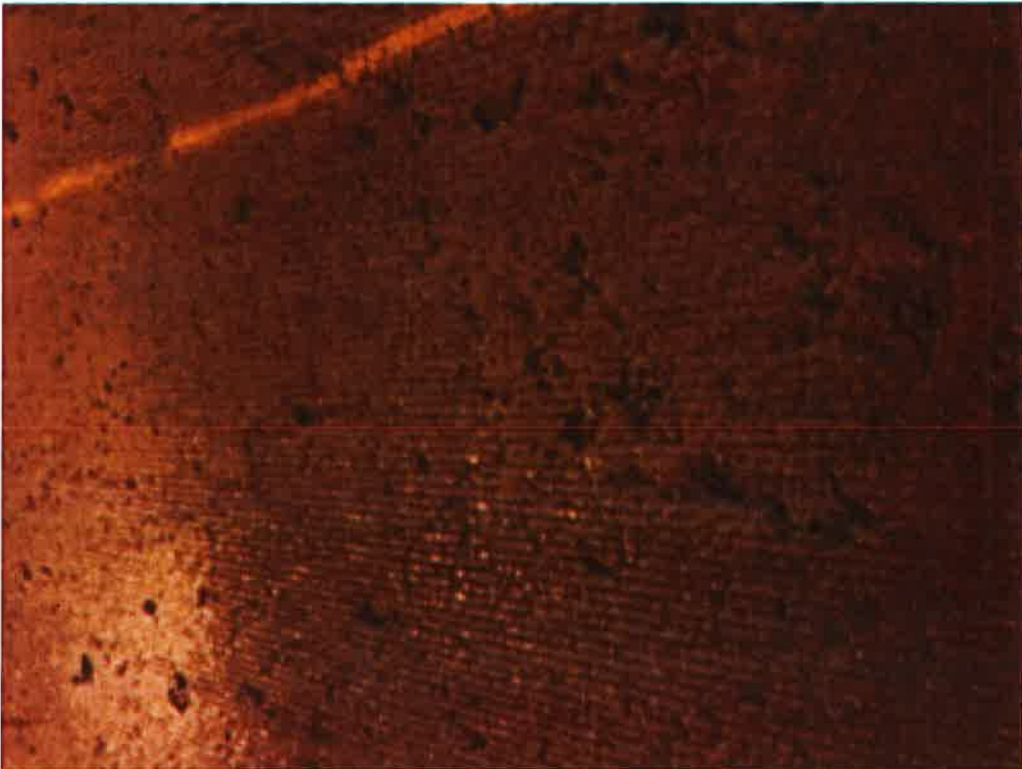
The Concrete Surface is polished in the Wheel Path; Course Aggregate is exposed
